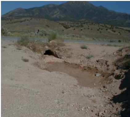
Photo 1. About 8% of the sub-watershed has severe to highly erosive soils.
