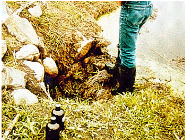
Improved Sinkhole Madison,
