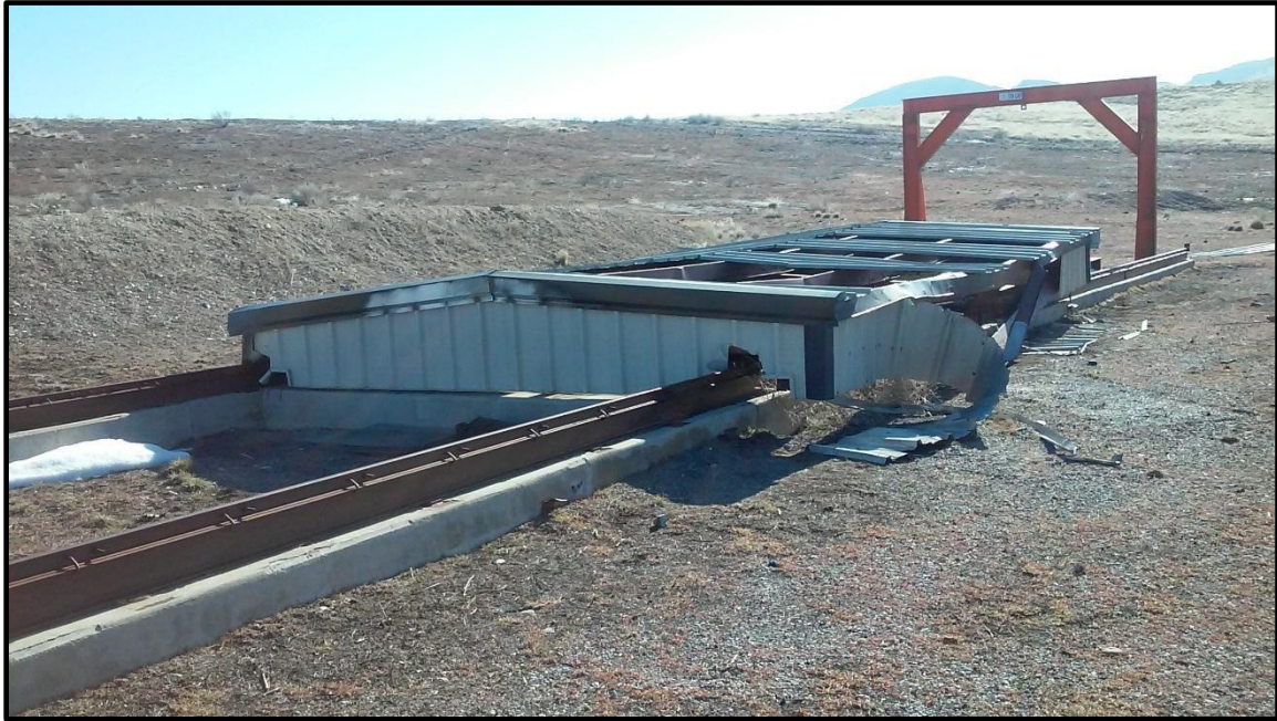
Figure 2. Burn pan showing weather cover and gantry (February 2017).
