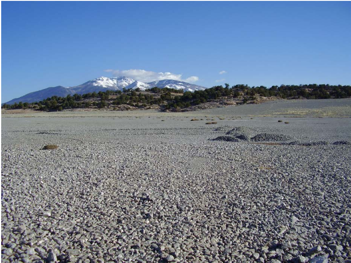
Photograph #2: The top of the Lower Tailing Impoundment. Showing the completed erosion barrier.
