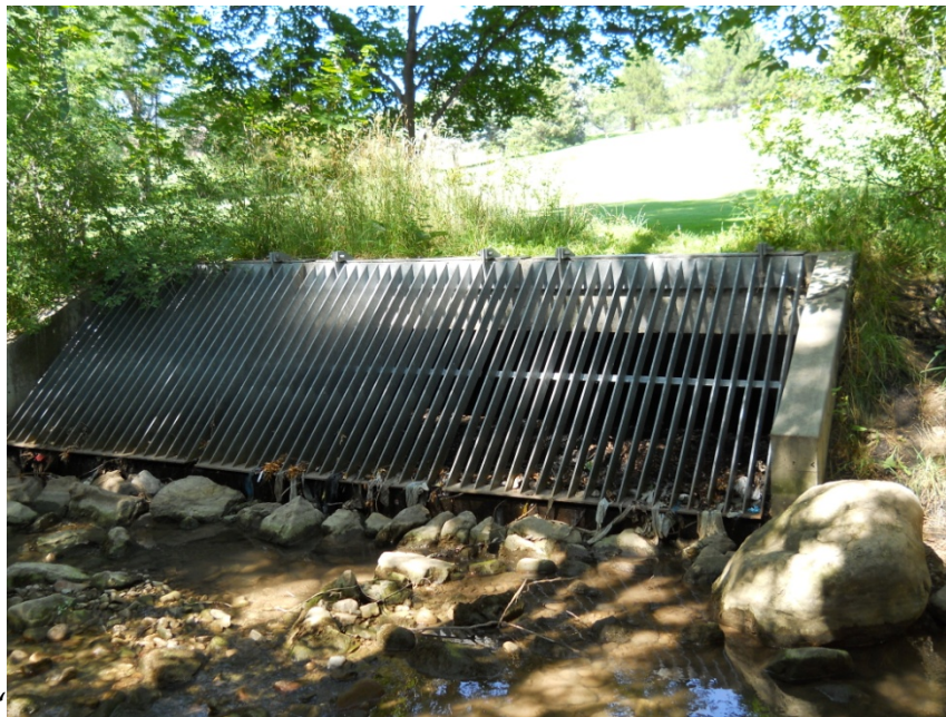
Photo 32: Parleys Creek below 1700 E, large outfall along north (secondary) channel, approximately 100-150 ft. downstream of 1700 E culvert outlet.
