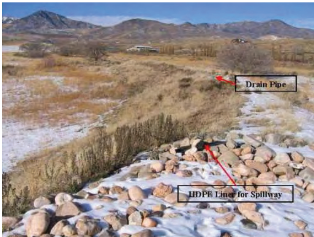
Photo No.16 – Top of the emergency spillway of the sedimentation basin of OU5, and along the northern embankment (in the near distance) is the vertical drainage pipe.
