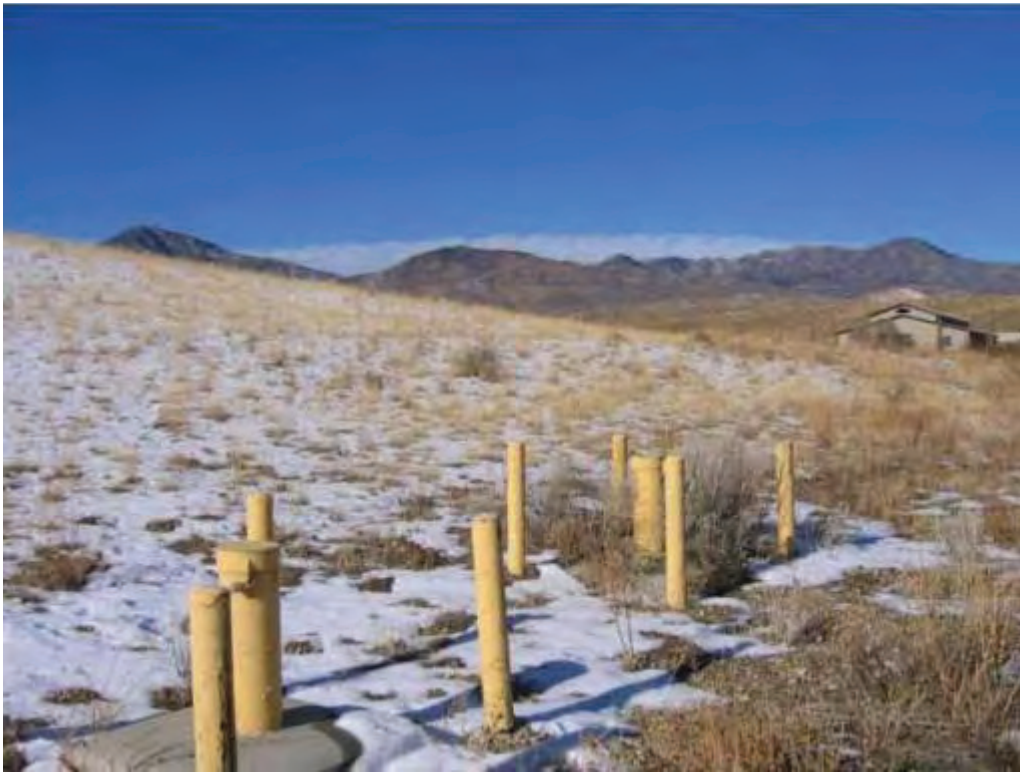
Photo No.19 – Monitoring wells, completed at different depths. These wells are located approximately at the northeast corner of the tailings repository at OU5.
