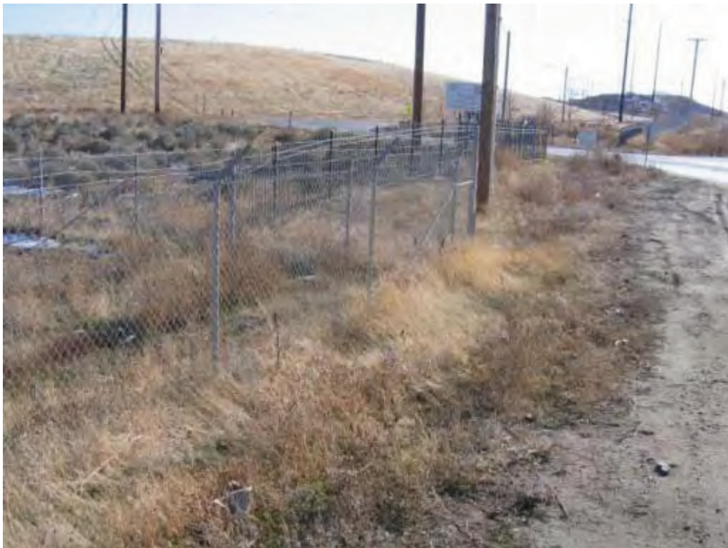
Photo No. 28 - Area of the repaired erosional cut along Rt. 111 as it is today.
