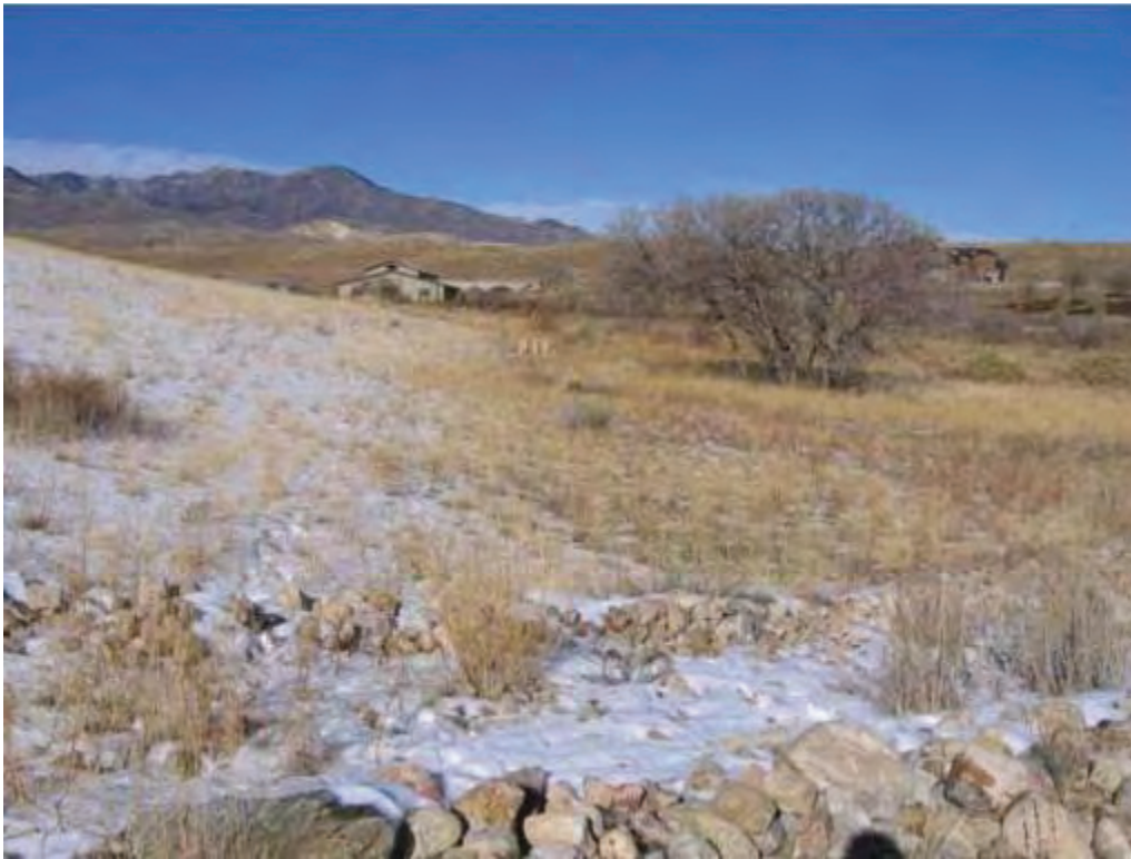
Photo No.21 – Southern run-off ditch as it straightens and heads north to connect to the north run-off ditch. This ditch is underlain by HDPE liner with rip-rap over the top.
