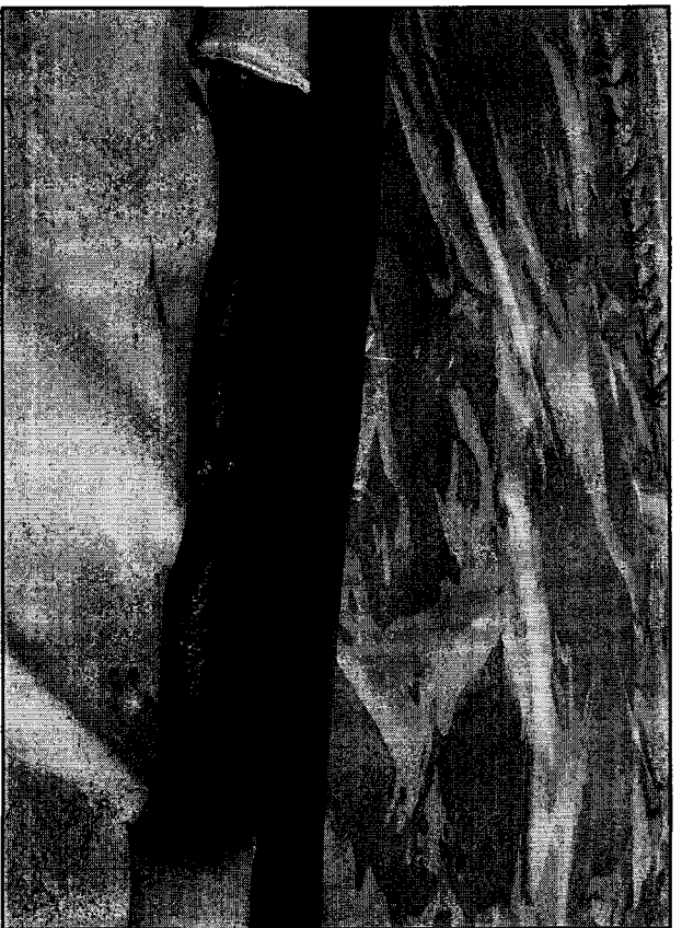
Photo 2. Connection of fabrics between sandbag ballast, slimes drain backbone. Note rock exposed, but not on the liner.
