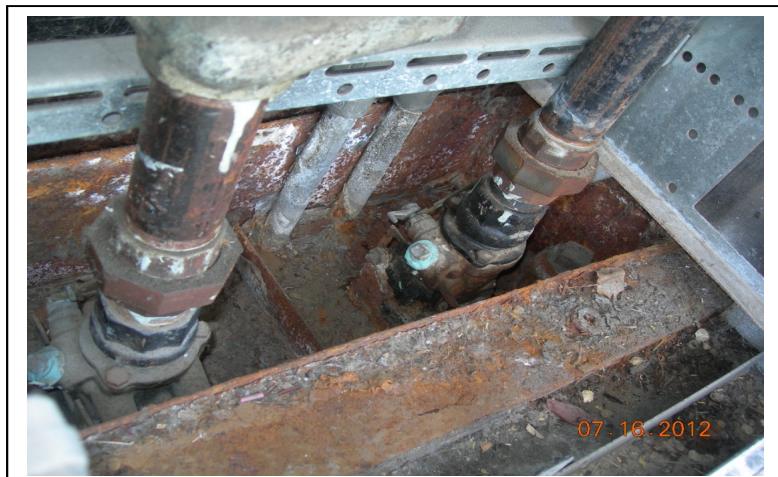
Sump Not Liquid Tight
